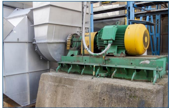
Large Centrifugal Fan -typically the fan drive and fan bearings are the components monitored. This fan does not have a backup.
