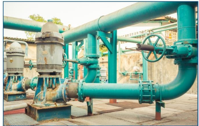
Vertical Water Pumps- pump drive and pump bearings are the components monitored. Loss of one pump could affect the ability to meet peak water demands.
