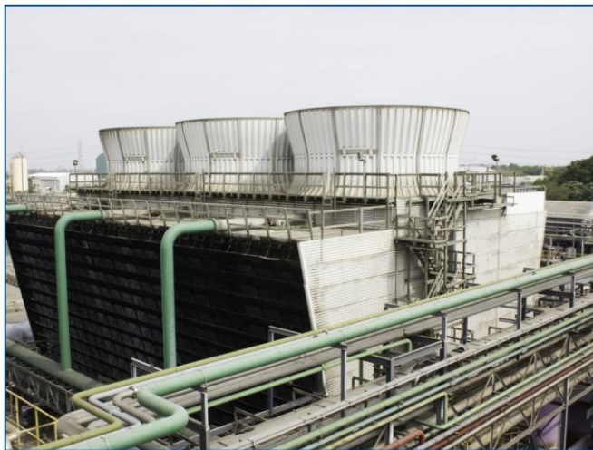
Cooling Tower Fans- typically the fan motor and gearbox are candidates for monitoring. Loss of a cooling tower fan gearbox could limit available cooling and reduce production capacity.
