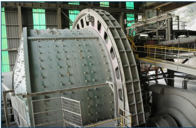
SAG and Ball mills at an ore processing facility- typically the mill drives, the mill gearbox and mill bearings are monitored. Loss of one SAG mill could result in a significant production shortfall.
