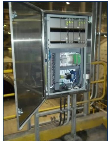
A 48-channel AMS 6500 deployed in a A6500PRE-SS-WM-/C wall mount enclosure, monitoring SAG and Ball mills at an ore processing facility
